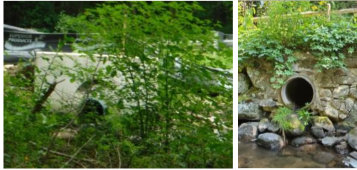
Figure 2-12. Examples of stormwater outfalls that discharge water in catch basins located on roadways and other impervious surfaces; their associated network of drainage pipes discharge stormwater away from the roadway and onto the ground or into a nearby river /stream.
